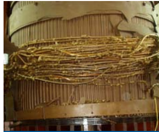
Collapsed tap winding
